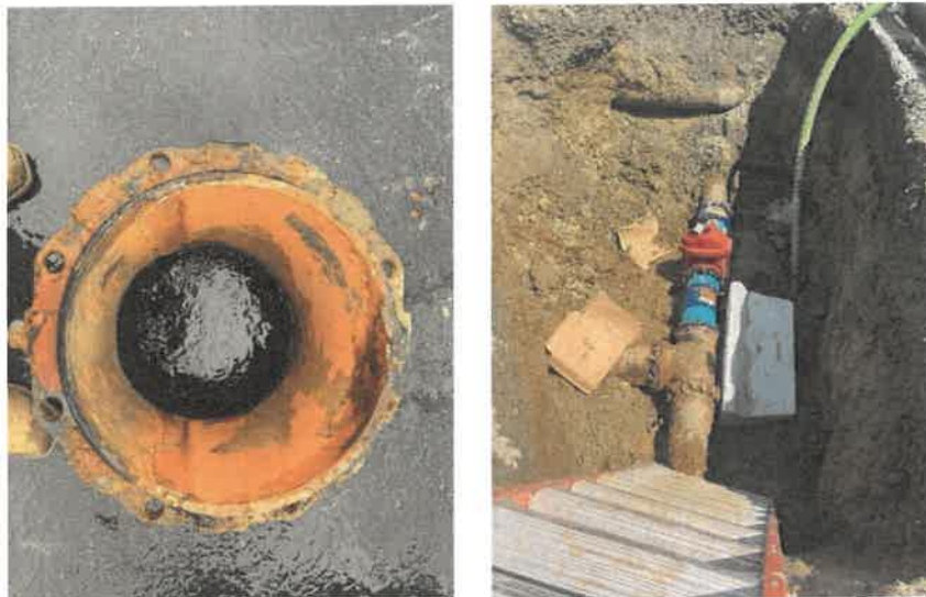
Figures 1 & 2: Pipe Corrosion and Repair
